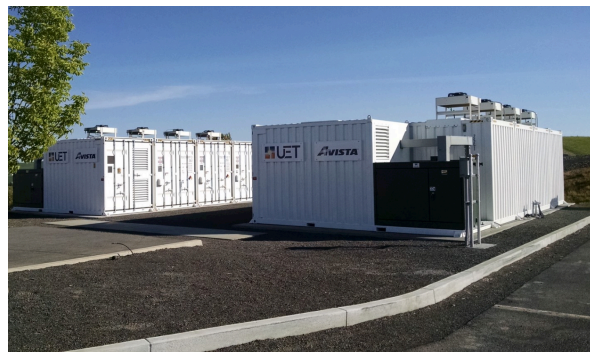
A 1 MW/4MWh vanadium flow battery operating in Pullman, WA PHOTO: Wikimedia Commons
